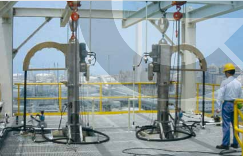
Installed lance systems over several floors for big strokes
