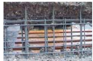
Concrete resurfacing and demolition with the URACA Vario Jet. The impressive demolition depth in hard concrete and the careful and efficient exposure of the reinforcement speaks for itself.
